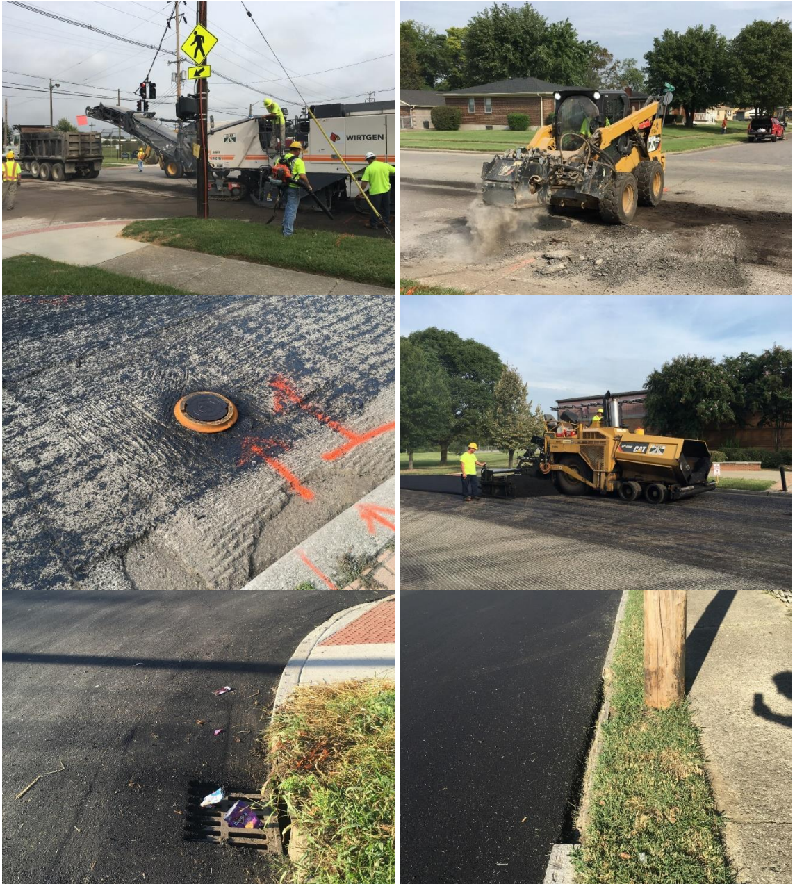
Fig. 5.7. Field view of mill and overlay on Southern Avenue in Louisville, KY
