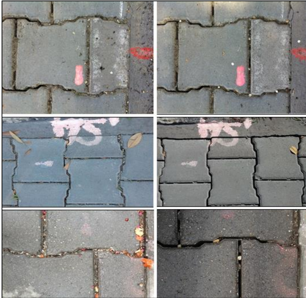
Figure 80 - Pre (left) and Post (right) Maintenance Photos. Sweeper/Vacuum Truck (top). Pressurized Airjet #1 (middle), and Vac-Head (bottom)
