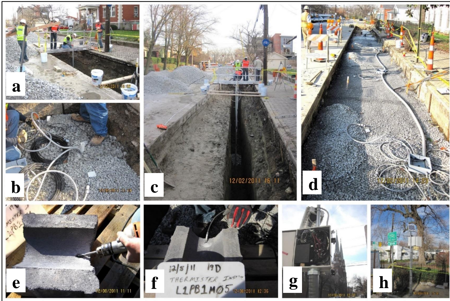
Figure 19 - Installing Sensors in Controls 19G & 19H: a,c) installing piezometer cluster and infiltration tests at the bottom of the trench were conducted from the spanning bridge b) installing surface TDRs d) wires were passed through flexible conduits e,f) thermistor installation g,h) data logger and enclosure
