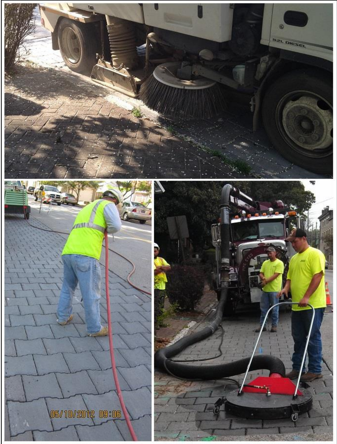
Figure 81 – The Three Methods Used for Restoring Infiltration Capacity of Controls 19G and 19H: Sweeper/Vacuum Truck (up), Pressurized Airjet (bottom, left), and Vac-Head (bottom, right)
