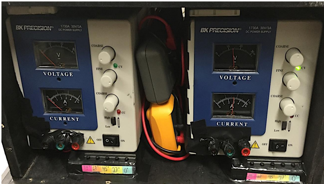
Figure 32. Upper Level Power Control Section
