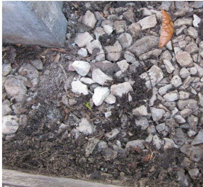
Figure 21. Sediment penetration into the storage gallery (a) Under paver blocks (b) Gravel layers
