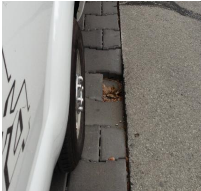
Figure 24. Block paver settlement (a) Adjacent to street pavement (b) Surcharge load
