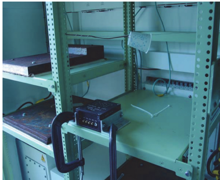
Figure 62. EDR mounting inside the rigid shelter (ATC Rail Impact Facility, 2005 approx.)
