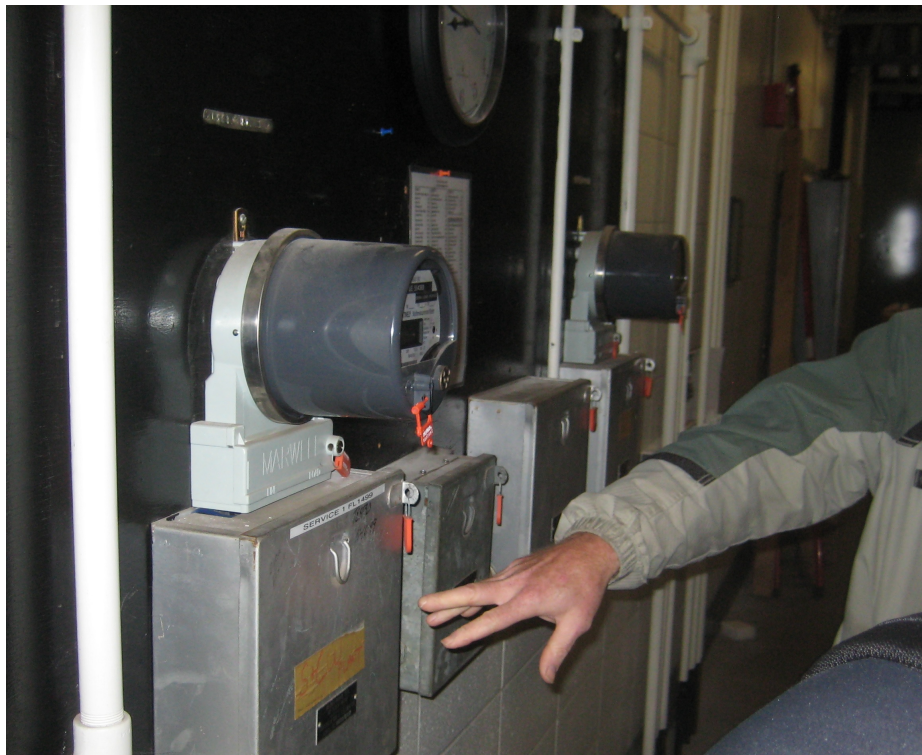
FIGURE 32: Louisville Gas and Electric utility meters installed on UofL Belknap campus.
