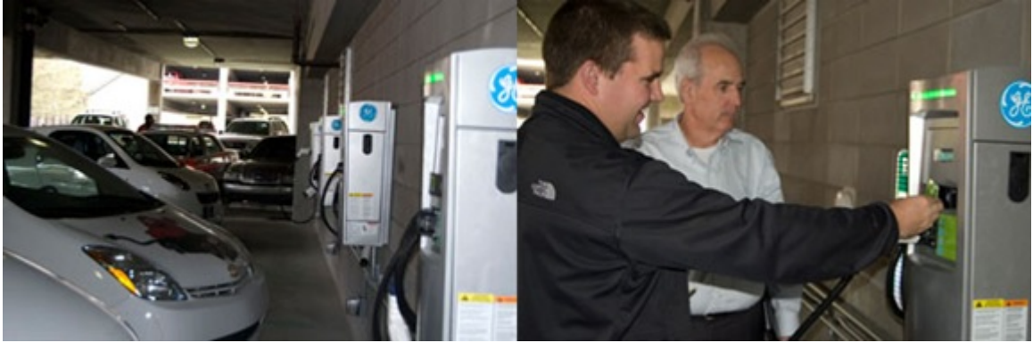
FIGURE 31: GE DuraStation level 2 EVSE installed on UofL Belknap campus [58].
