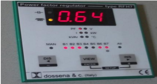
Figure 5.1: Capacitor stages C4, 5 are out of service.
