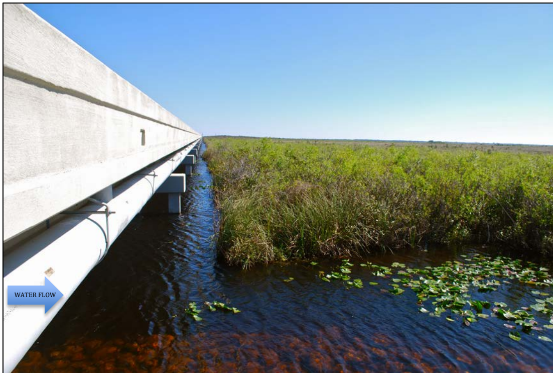
Figure 1.1: The LRR Bridge on Tamiami Trail (construction: 2010-2013); enhancing water flow south into the ENP by allowing flow under the east-west barrier of Tamiami Trail.
