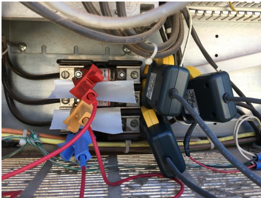
Figure 4-17 - power meter installed on the power supply to the VFD.
