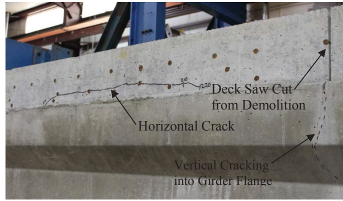
Figure 64 – Test D-5, Horizontal Shear Cracks
