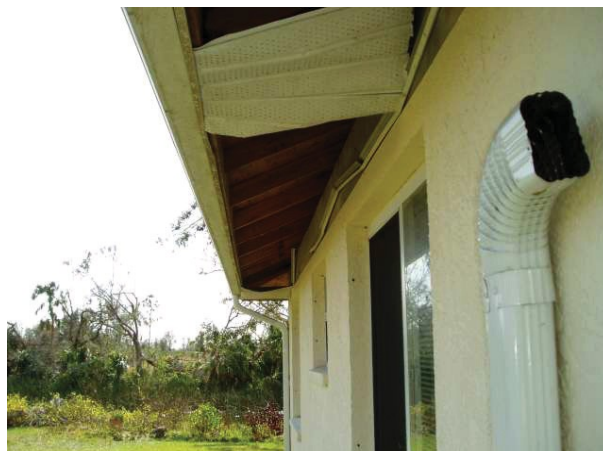
Figure 1-4. Damaged soffit due to wind-induced suction (FEMA)
