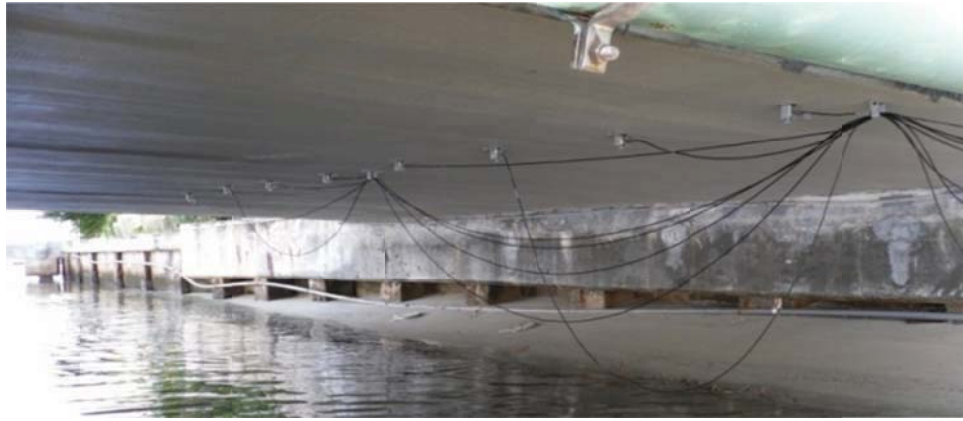
Figure 2.12 - AE sensors on deck soffit of the bridge
