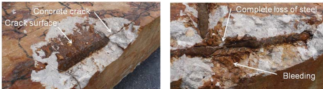
(a) Crack in concrete cover with bleeding surface
