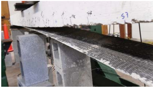
(a) Delamination B1
