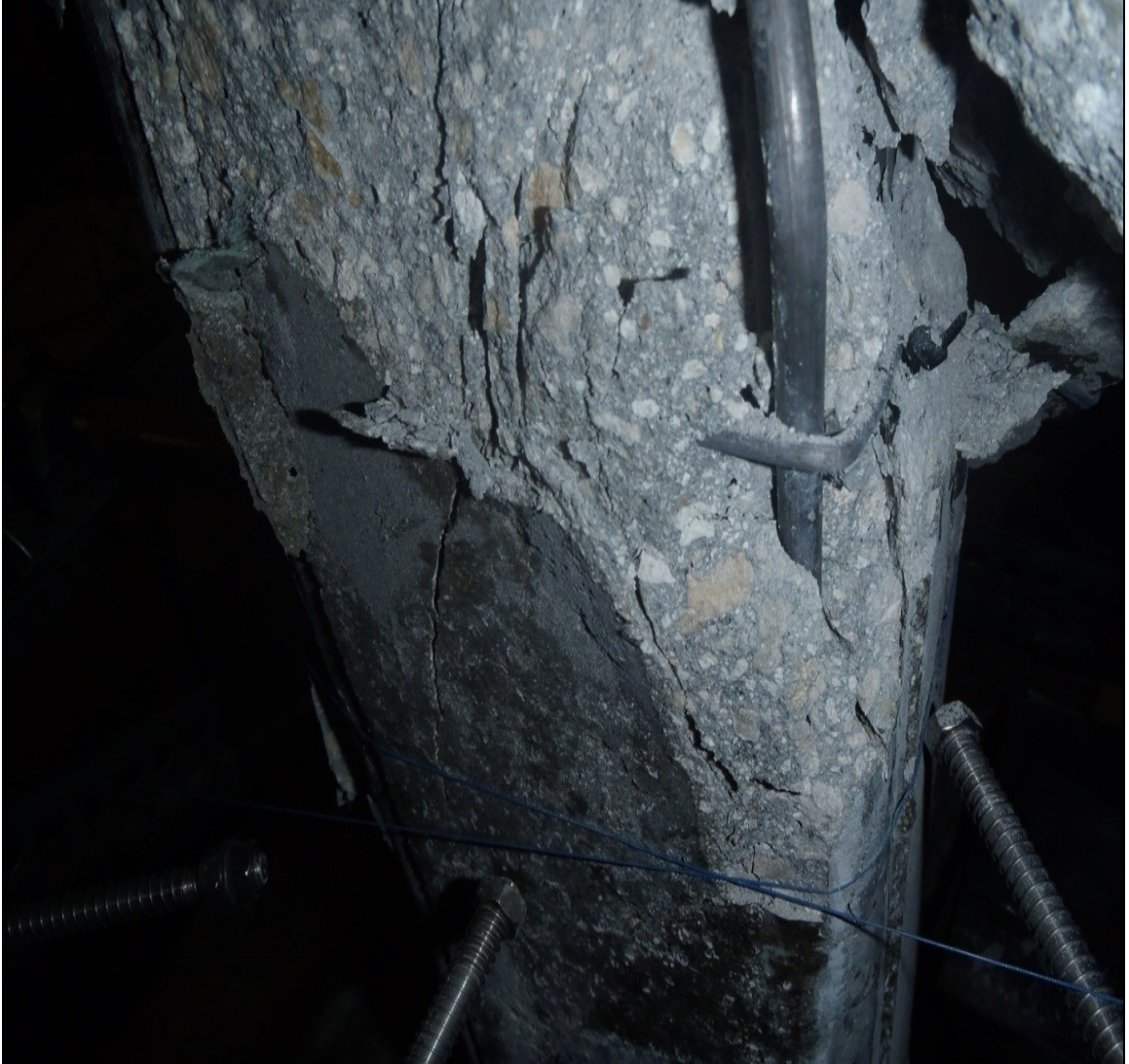
Fig. B-15: Failed control column
