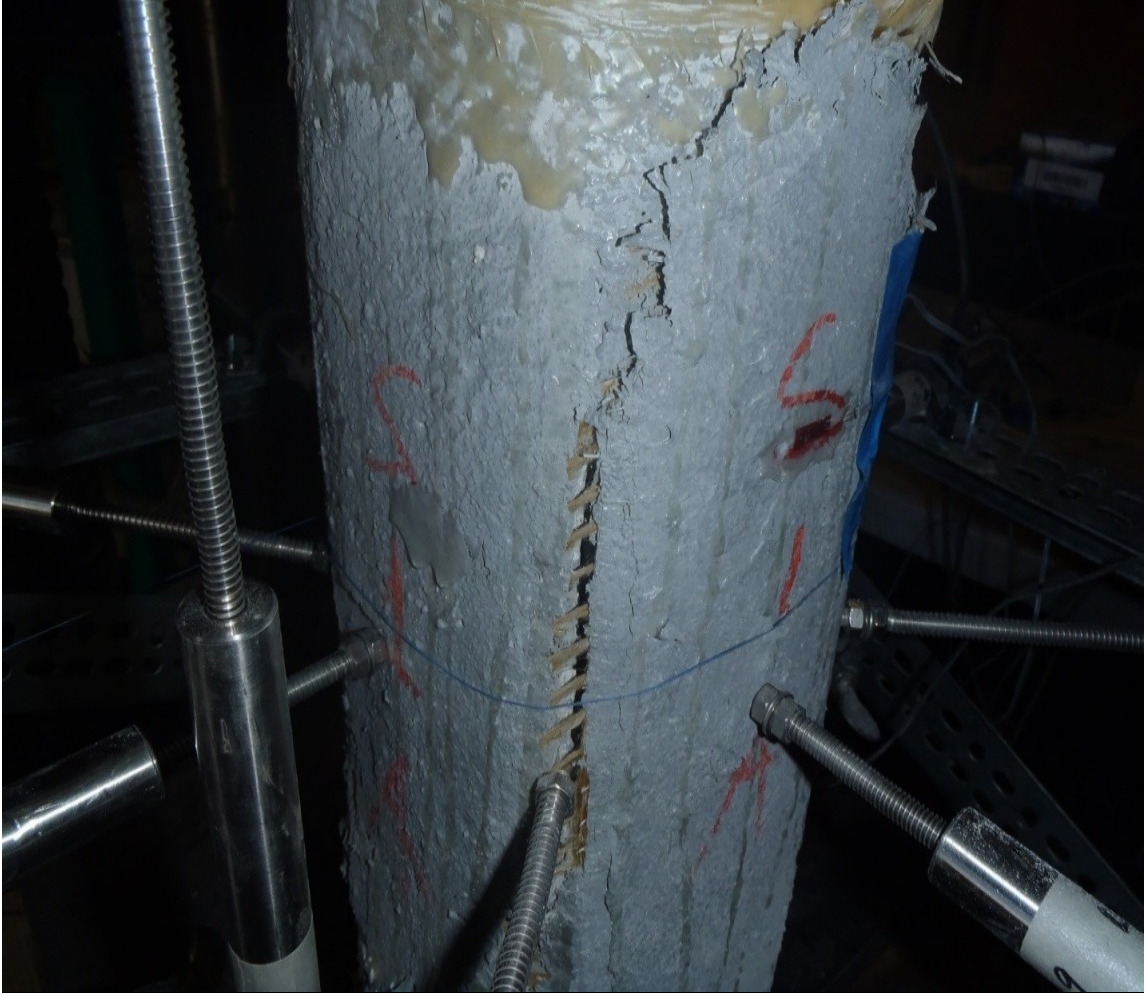
Fig. B-13: Failed PBO-FRCM wrapped square column
