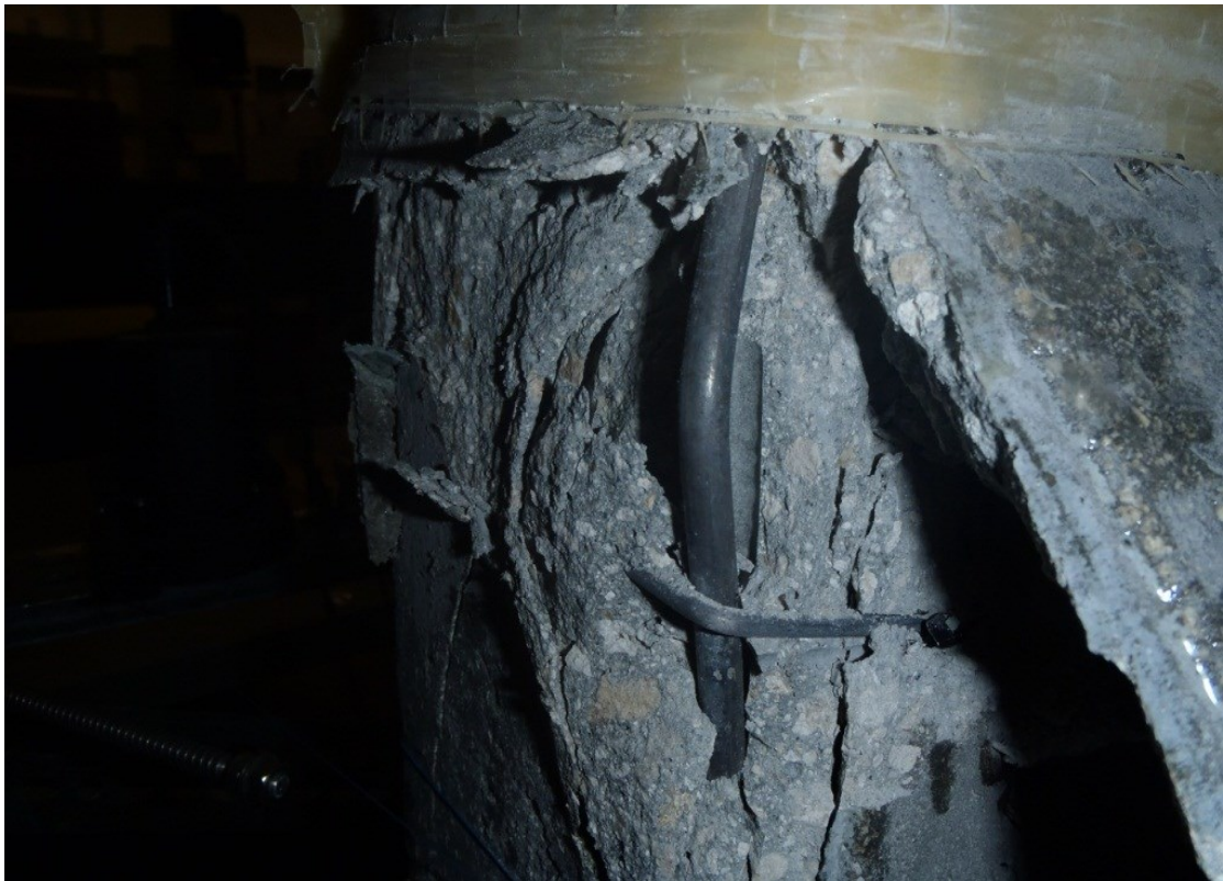
Fig. 4-5: Buckling of the internal steel reinforcement in RC column
