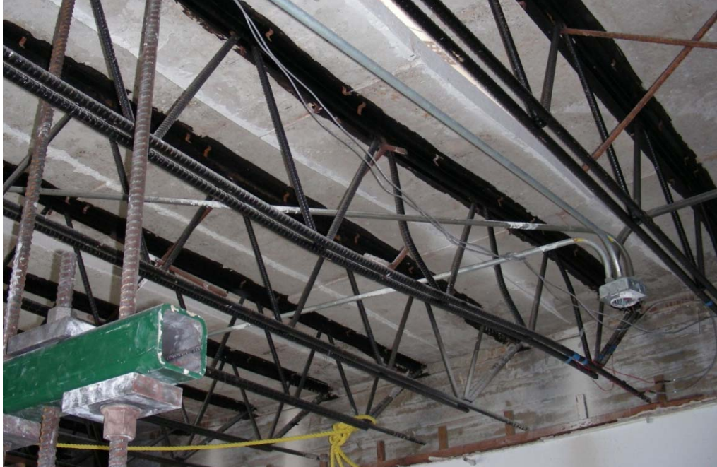
Figure 80 – Buckling Failure: Specimen No.2
