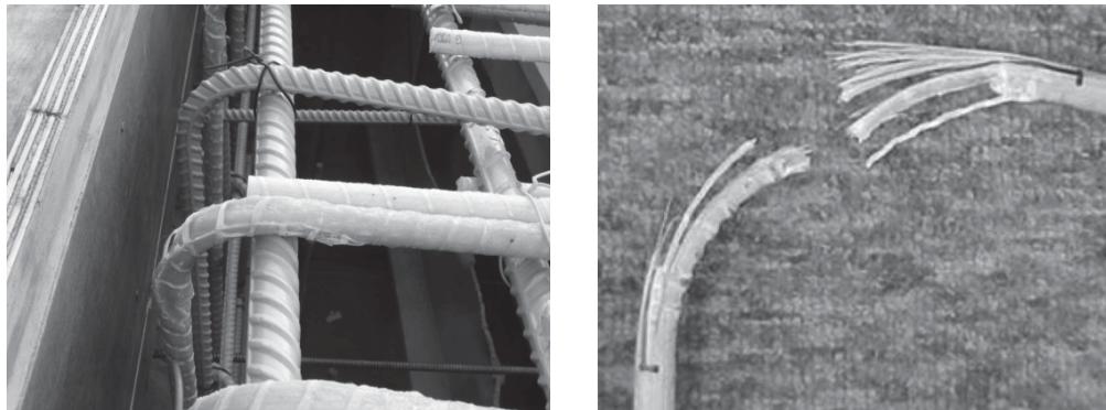
Figure 1.4 - (a) Bent bars in I-635 bridge deck over State Ave. in Kansas City (b) typical failure mode of a bent GFRP.
