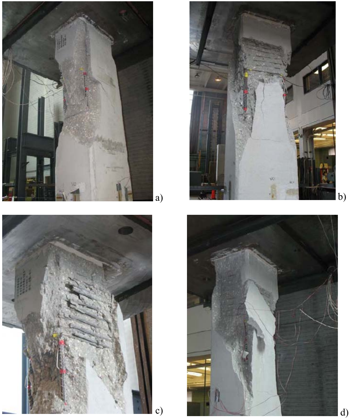
Fig. A - 29: Failure of Specimen R-0.5-control (a-d).
