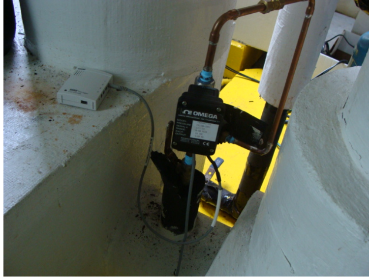
Figure 5.7: Differential pressure transducer for head measurement at pump discharge.
