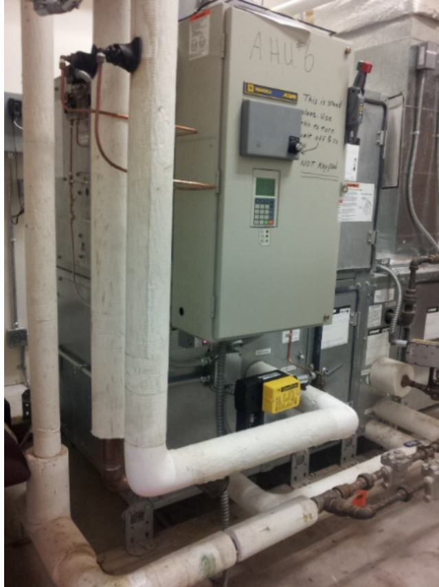
Figure 4.2: Air Handling Unit used in the experimental test site
