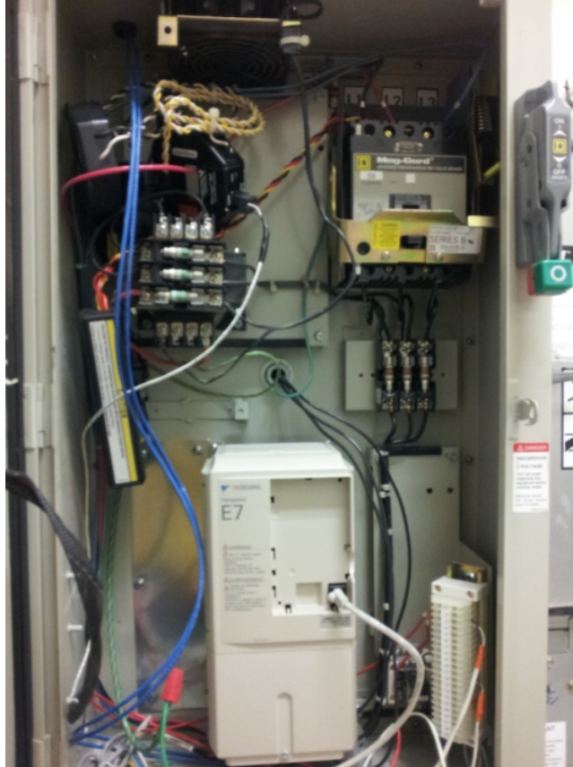
Figure 4.3: VFD installed on Fan Motor
