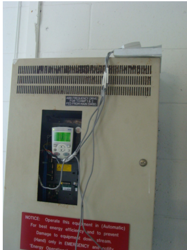
Figure 5.4: Motor input power and frequency measurements from VFD output panel
