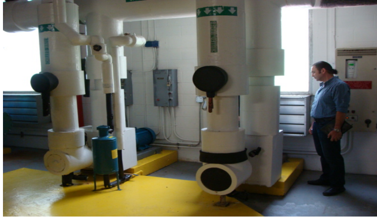
Figure 5.3: Chilled water pumps at the experiment site.
