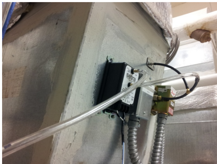
Figure 4.8: Differential pressure meter installed on ductwork
