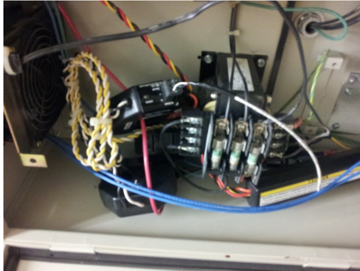
Figure 4.7: Power Meter installed upstream of VFD
