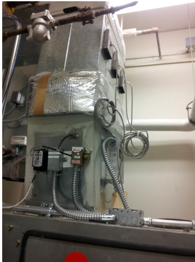
Figure 4.6: Air Flow Station installed in duct
