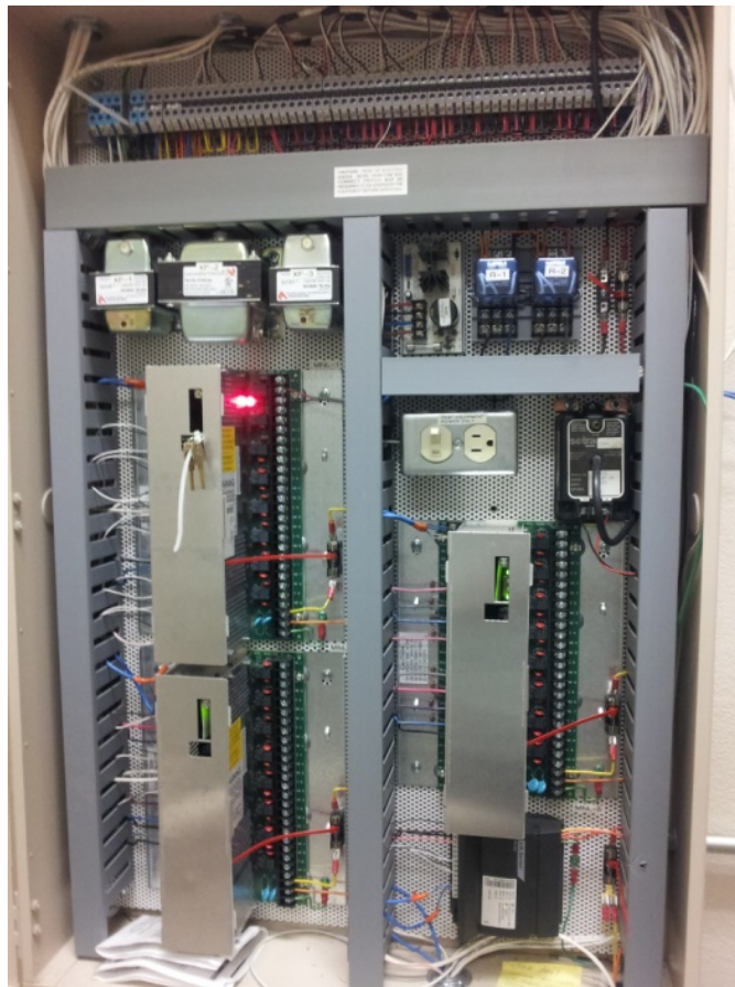
Figure 4.5: EMS Control Panel
