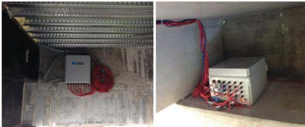
Figure 1.3: Data acquisition stations installed permanently below the Fate (left) and the Innovation (right) Bridge
