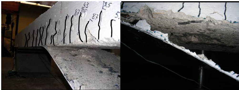
Figure 4.2 – Debonding failure exhibited by the specimen EB
