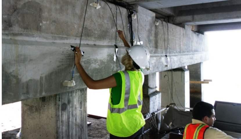
Figure 9 – Field SHM set-up of RC pier cap slated for repair
