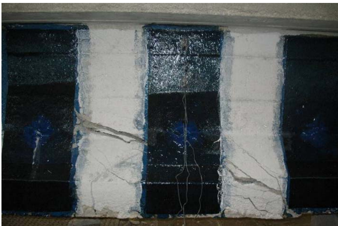
Figure 7.34 – B-4a Failed Section
