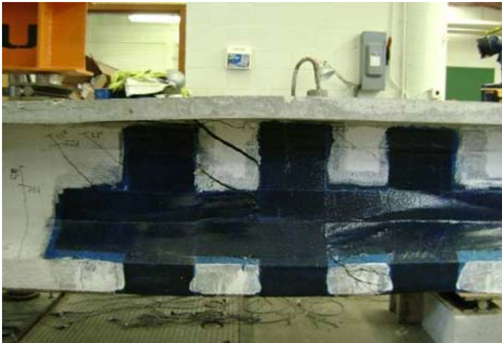
Figure 7.25 – B-3a Failed Section 1
