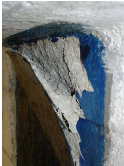
Figure 7.9 – B-2a Peeling of Laminate
