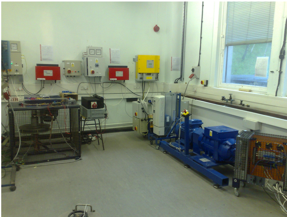
Figure 2.2: Photograph of Durham Experimental Small-Scale Energy Zone facility
