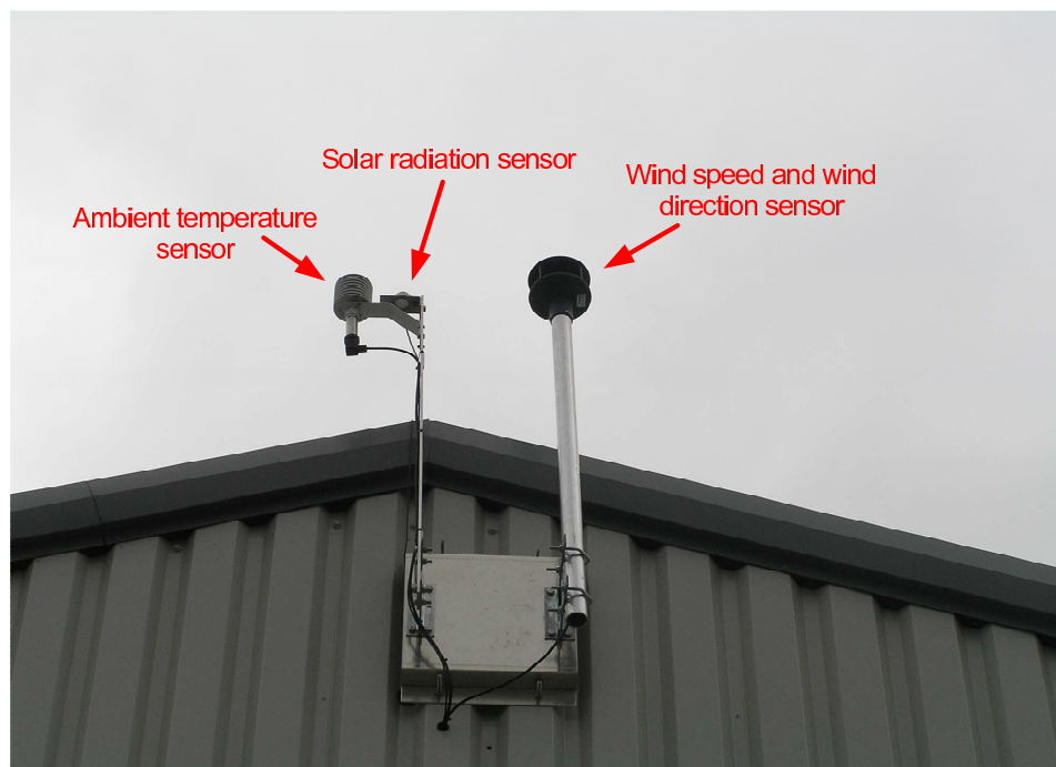
Figure 13.2: Meteorological sensors installed in the Rhyl substation compound
