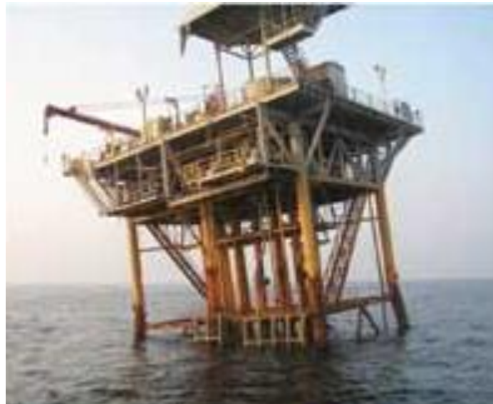
Figure 1.2: Collapse of platform due to hurricane www.offshore-mag.com
