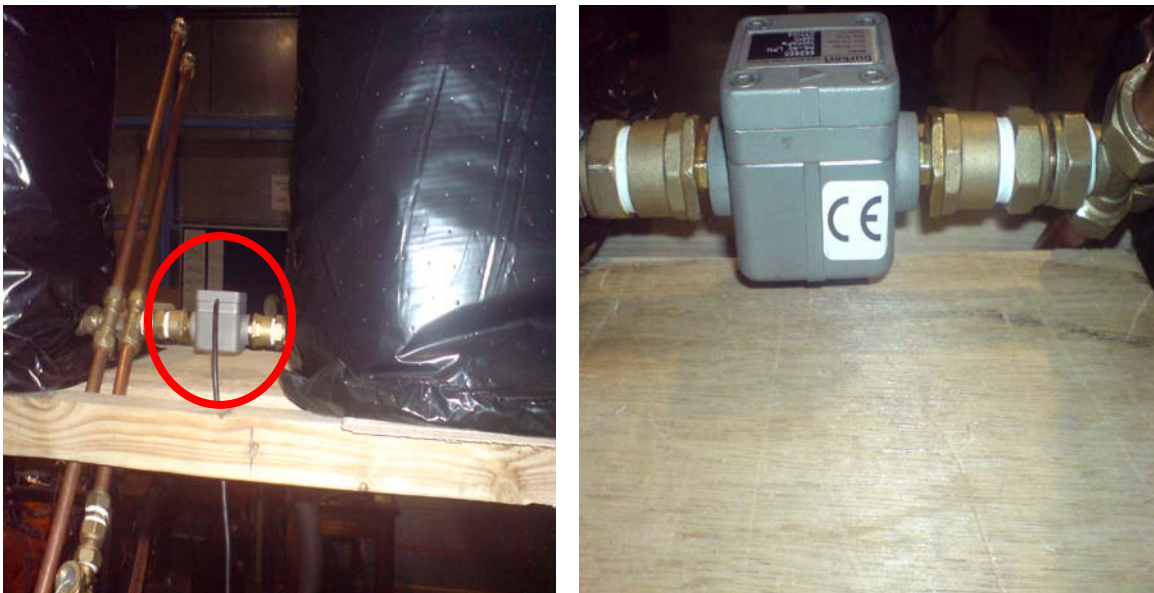
Figure 6.4g Mass Flow meter.
