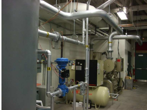
Figure 4.17: Piping for Air Delivery System
