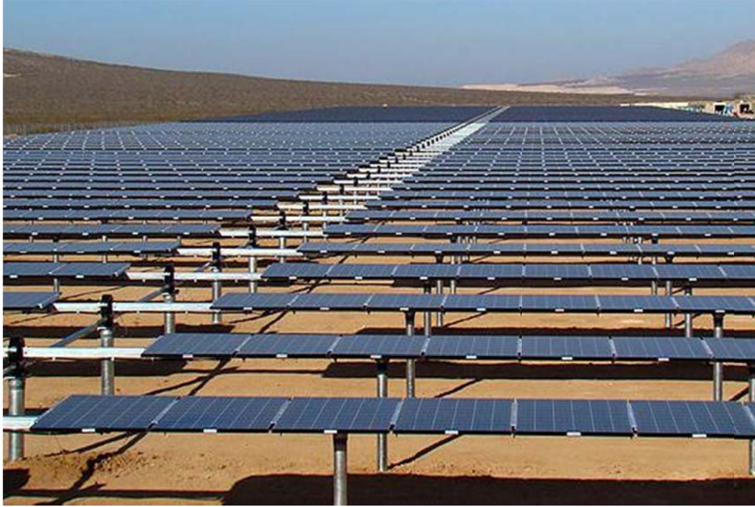
(c) PV array system
