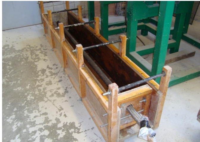
Figure 3.1: Photograph of 300 \times 300 formwork with H50 bar in position ready for casting.
