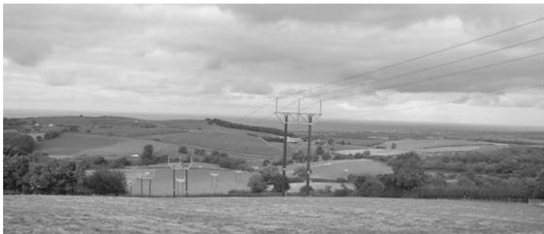
Figure 56: 132kV overhead line in the site trial area
