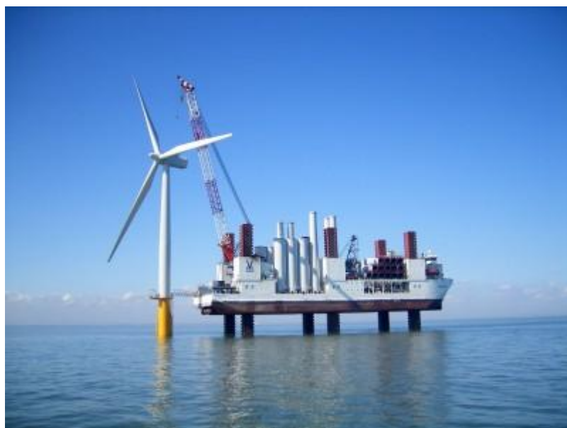
Figure 29: Example of a Mobile Fixed or Jack-up installation as used during the construction of Horns Rev and Kentish Flats wind farms.
