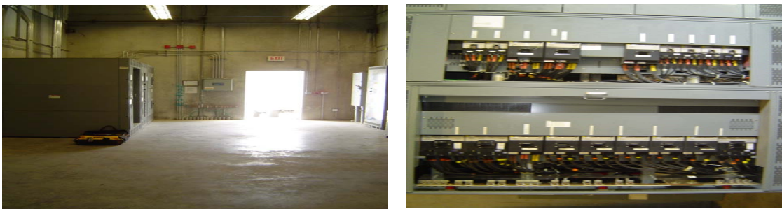
Figure 8: Main electrical meter room at the private company considered in this study
