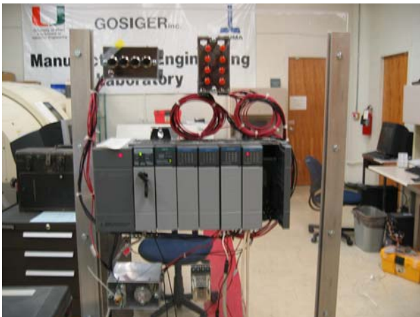
Figure 3-15 The Allen Bradley PLC (SLC 500) used in the Experiment
