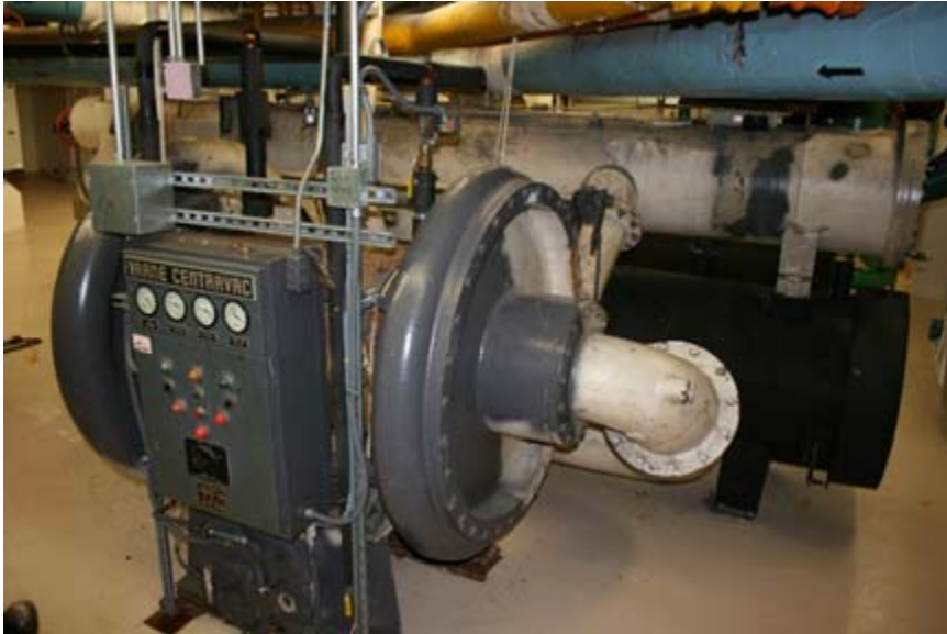
Figure 3-2 200-ton centrifugal chiller.
