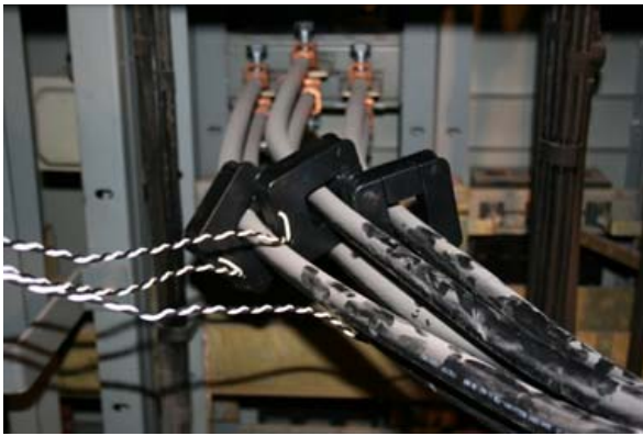
Figure 3-19 400 amp current sensor transformers phases a,b,& c..
