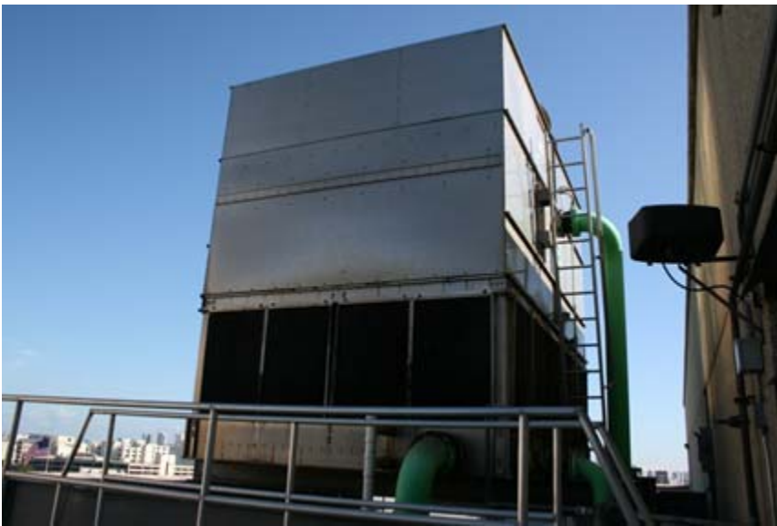
Figure 3-5 200-ton HVAC cooling tower.
