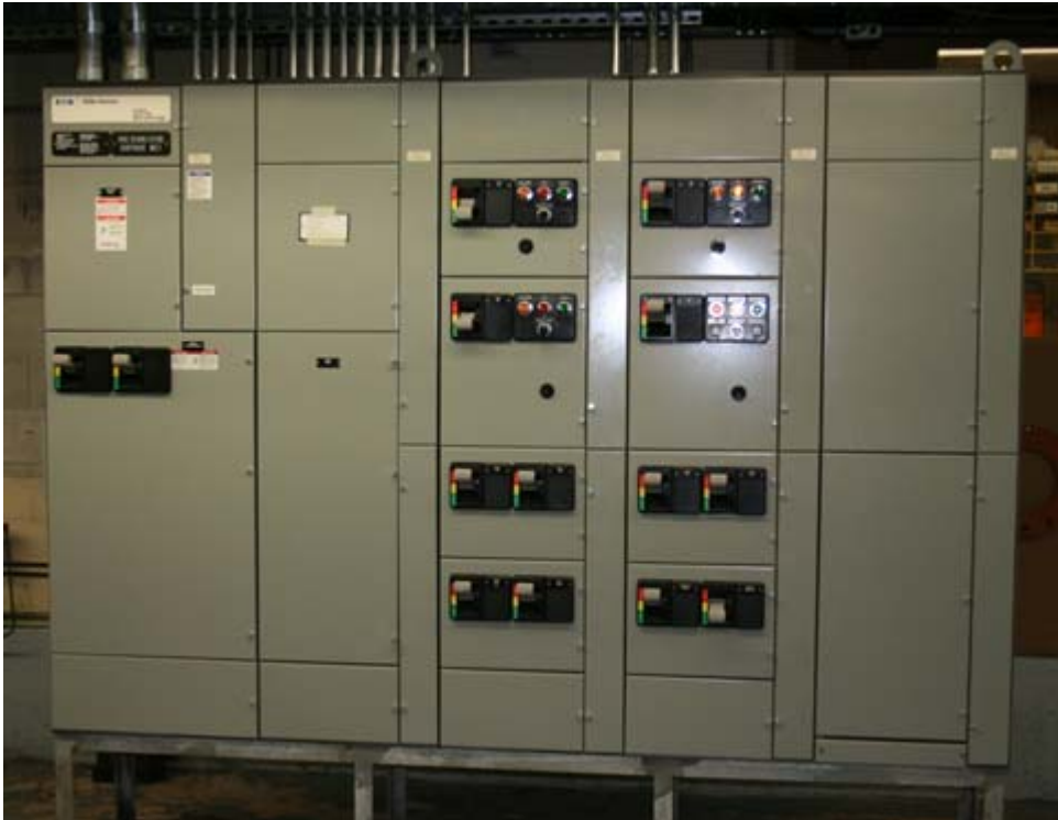
Figure 3-14 – Motor Control Center #1 (480V, 600amp).
