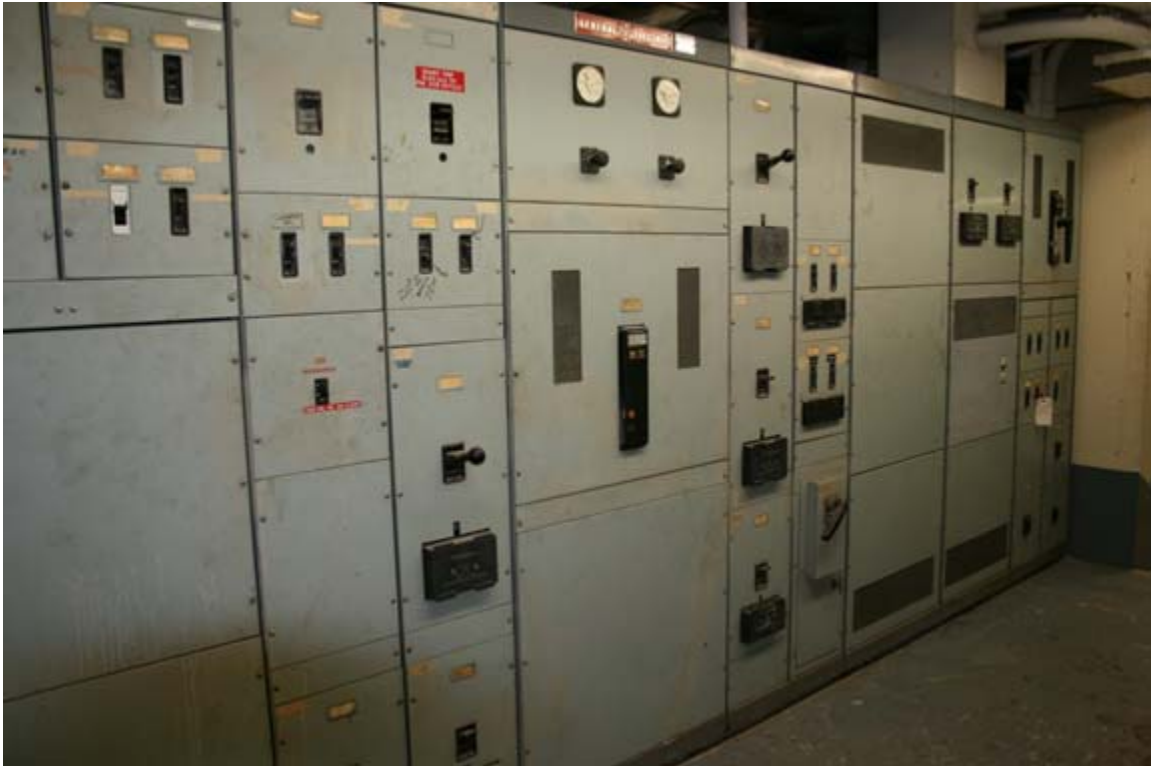
Figure 3-9 – Main Service Entrance #1 (480V, 3000amp).
