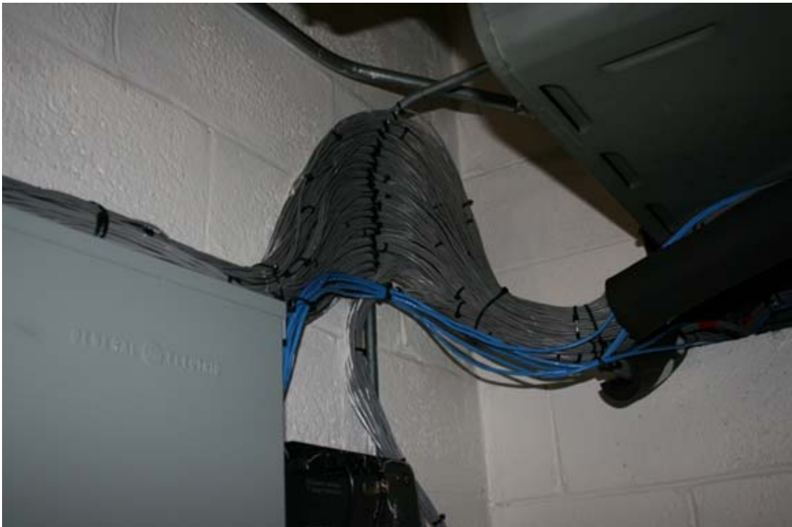
Figure 3-26 Sensors and communications cabling.
