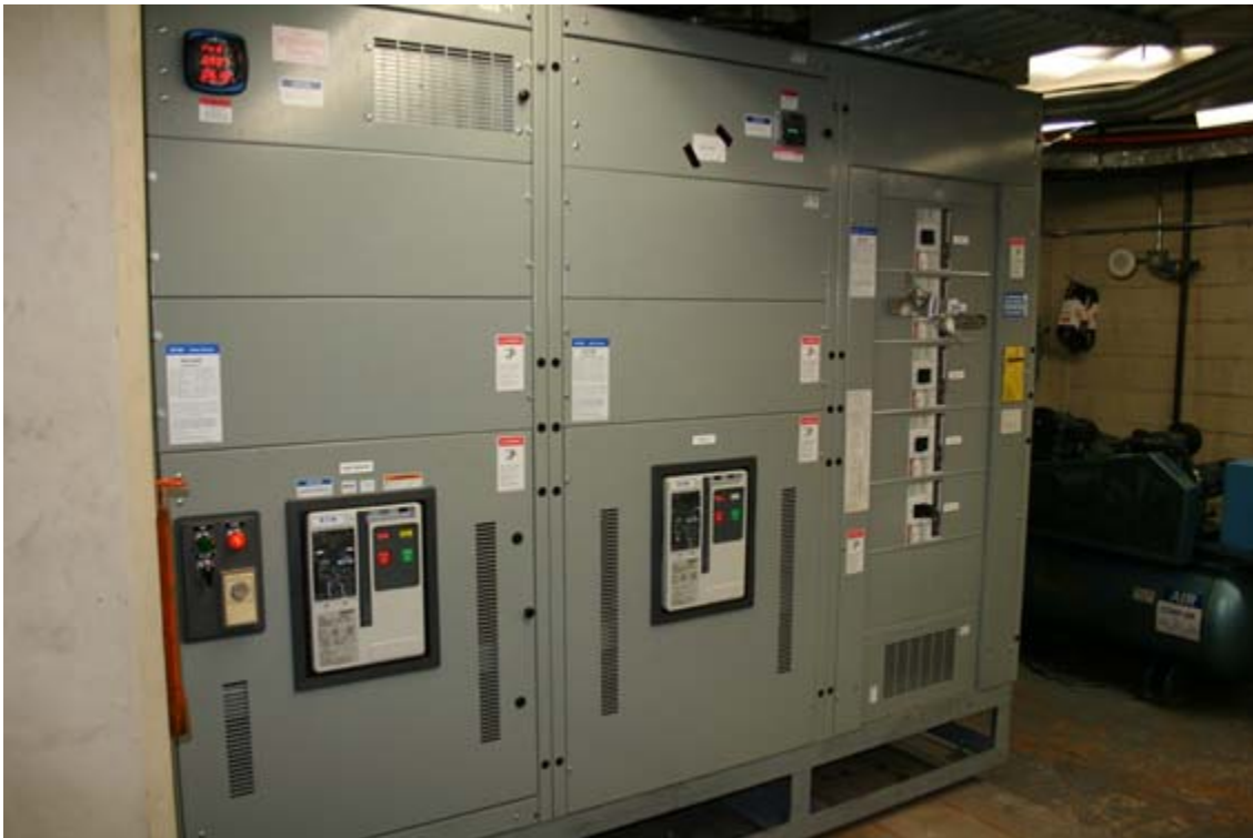
Figure 3-11 – Main Service Entrance #2 (480V, 3000amp).
