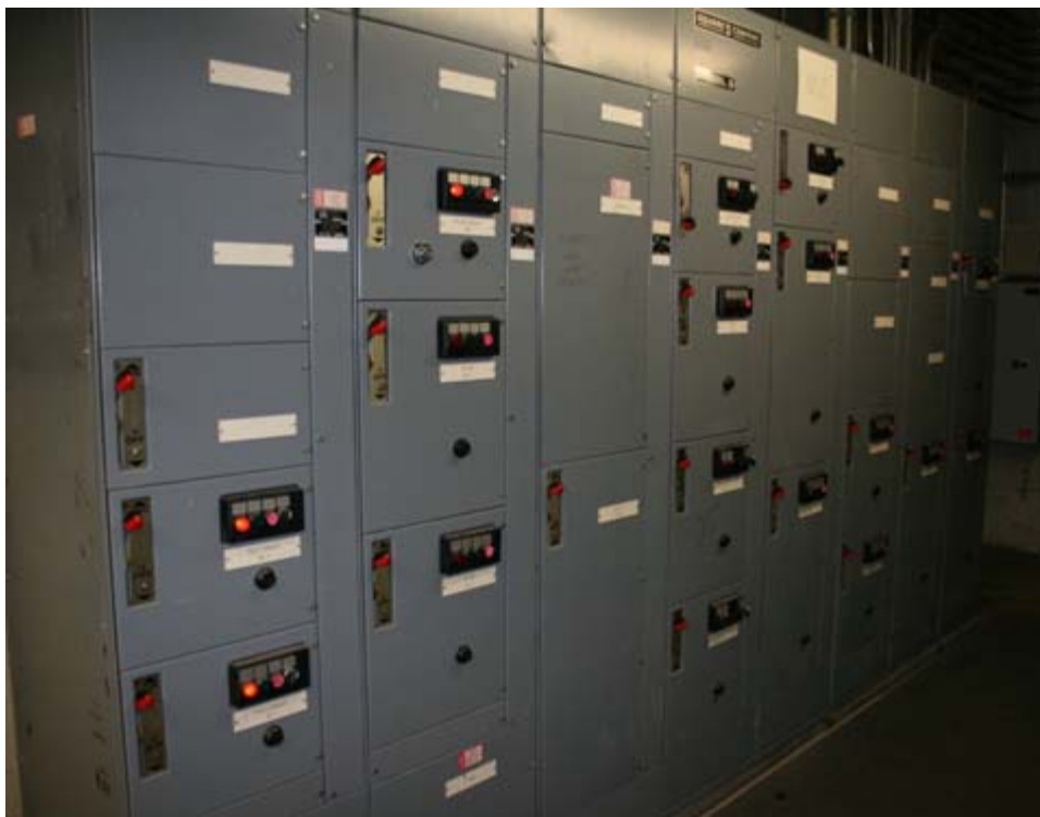
Figure 3-16 – Motor Control Center #2 (480V, 1600amp).
