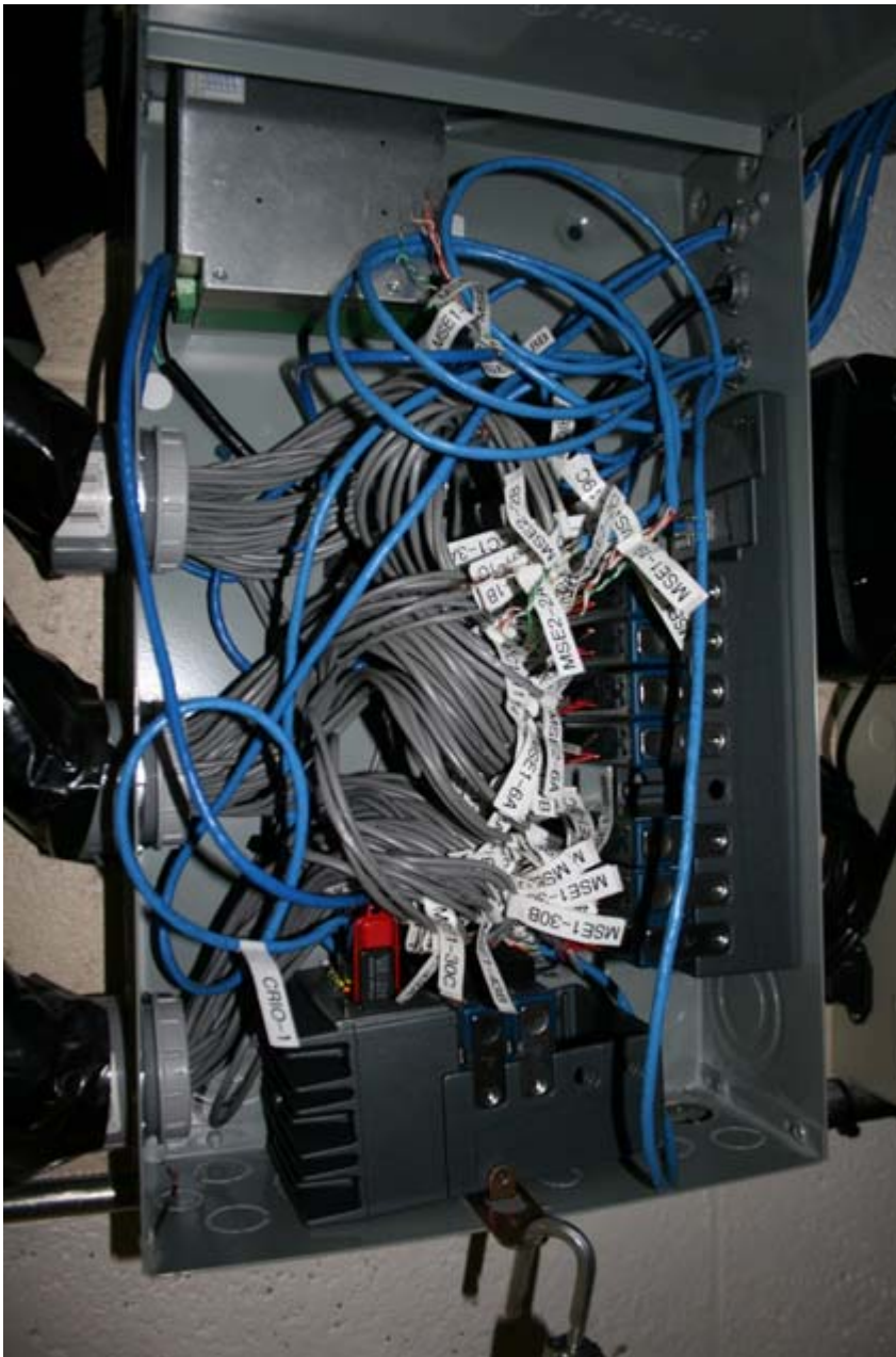
Figure 3-25 National Instruments hardware control box with cRIO and EtherCAT.
