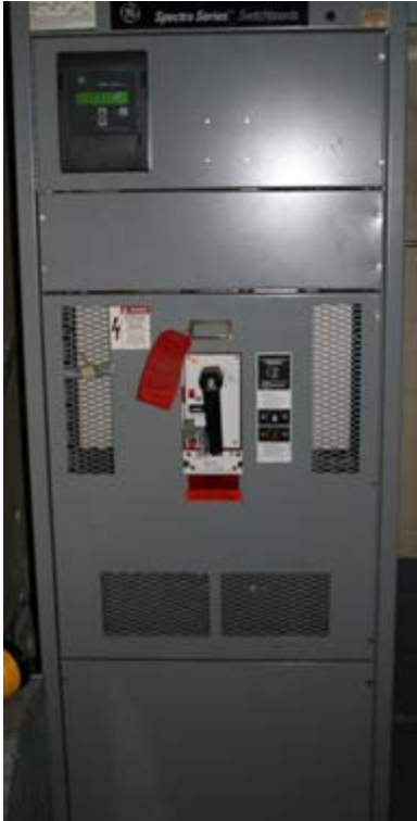
Figure 3-13 – Main Service Entrance #3 (480V, 1200amp).
