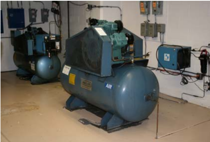
Figure 3-7 4 x 7.5 HP air compressors.
