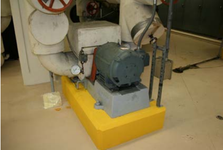
Figure 3-4 25 HP chiller pump motor.
