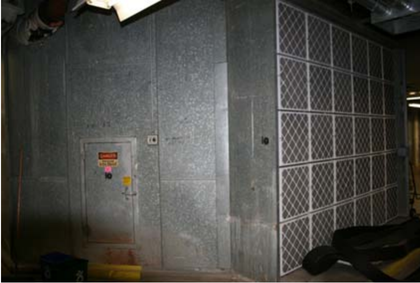
Figure 3-6 75 HP HVAC air handling unit.
