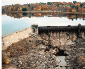
A visible disjuncture on opposing sides of the Turners Falls Dam
