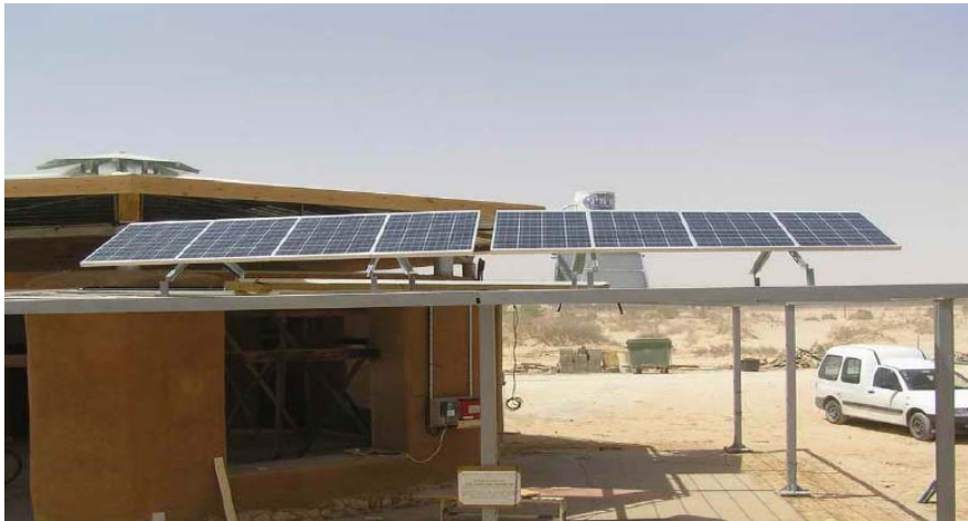
Fig. (6.1) Photovoltaic unit in a village in the West Bank
