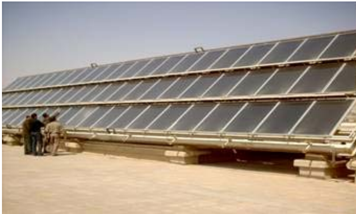
Fig. (3.4) Collective Solar system at Jericho hospital Source; www.perc.ps
