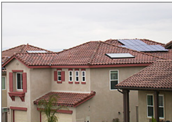
Fig. (3.5) Direct pump system on the roof of villas
