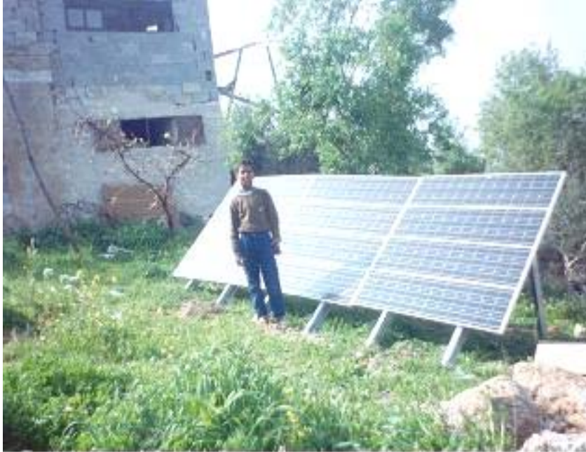
Fig. (3.13) PV array in one of the village
