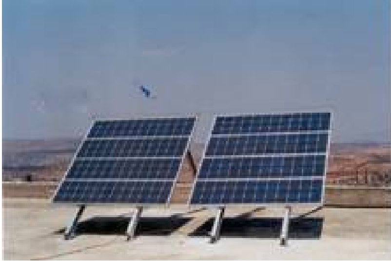
Fig. (3.16) PV system, rural clinic- Kufor Thulth village in the north of West Bank.
