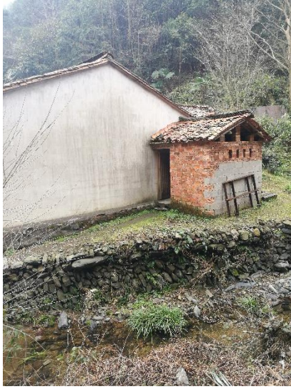
Figure 37 The addition looks inharmonious with the existing building
