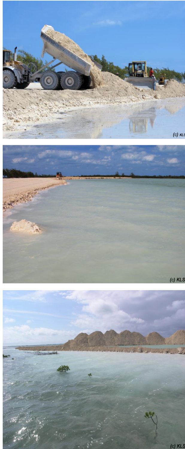
Figure 3.2. Construction activity within the North Sound, Bimini, Bahamas. Top: Fill material is dumped on the shoreline with no sediment mitigation barriers. Middle: Fill material is transported to an area deforested of mangroves and deposited along the shoreline. Bottom: Mounds of excavated fill material are piled behind a deep dredge pool in an area that had previously been a mangrove forest wetland. Plumes of sediment can be seen flowing into the nursery in the middle and bottom images.
