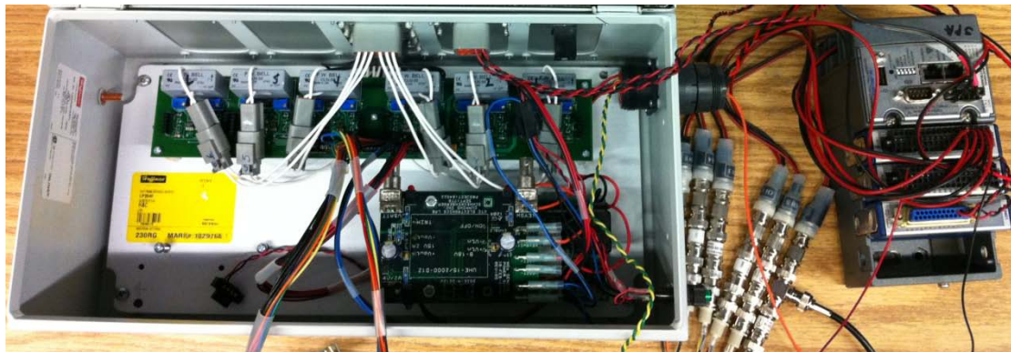
Figure 3.7 Hardware to capture the injection signal
