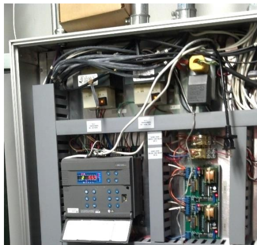
Figure 4.7 Original DX controller responsible for AHU controls
