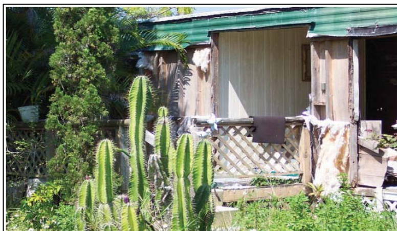
Figure 4.15. Abandoned Mobile Home, Source: Keef59, Flickr.com Used with permission.
