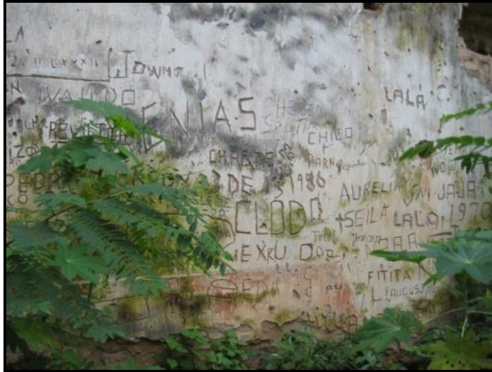
Figure 7.25: Human markers on the walls of the church ruins
