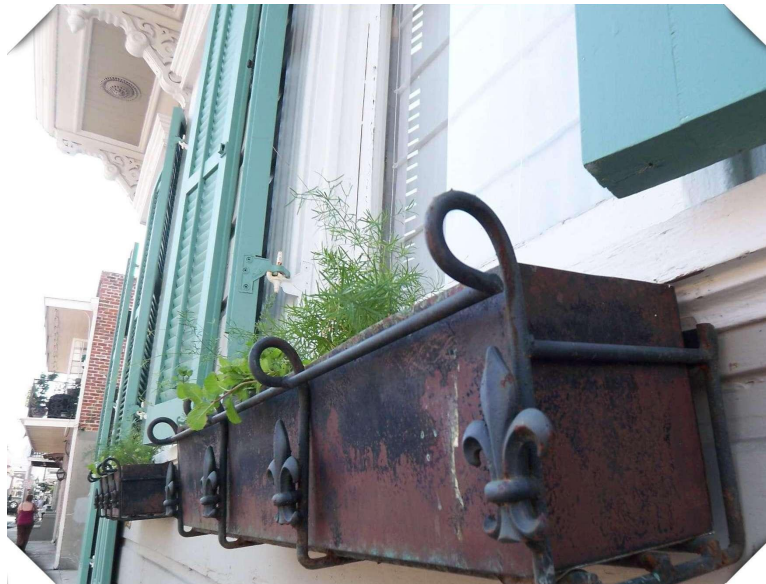
Figure 18 Detail of a House in the French Quarter; source: photographed and processed by author
