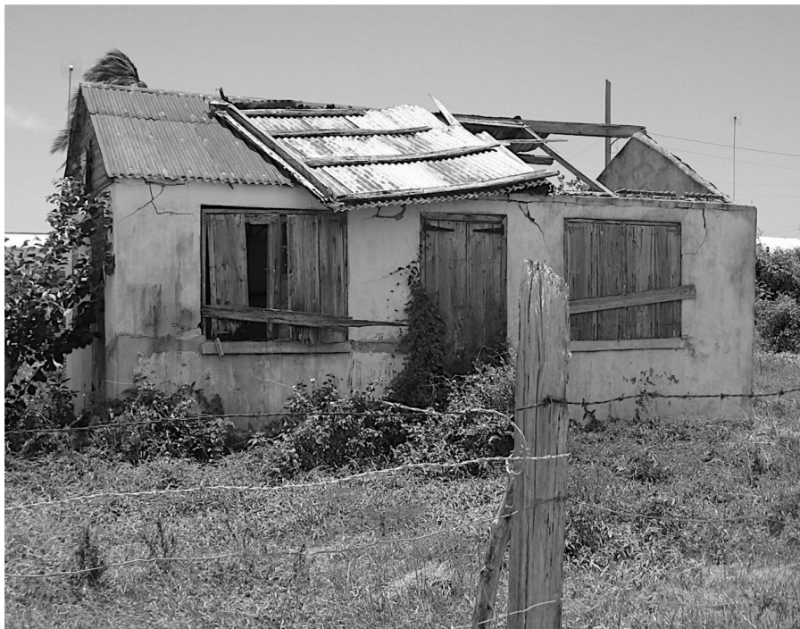
Figure 3.10 One of many abandoned homes throughout the village.
