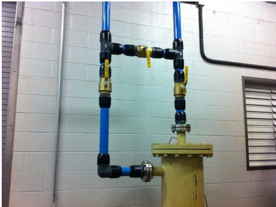
Figure 2-6: Mist eliminator filter and associated piping. Photograph by A.C. Harding, used with permission.
