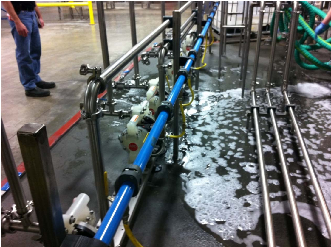
Figure 2-4: Diaphragm pump header regulated to 55 psig. Photograph by A.C. Harding, used with permission.
