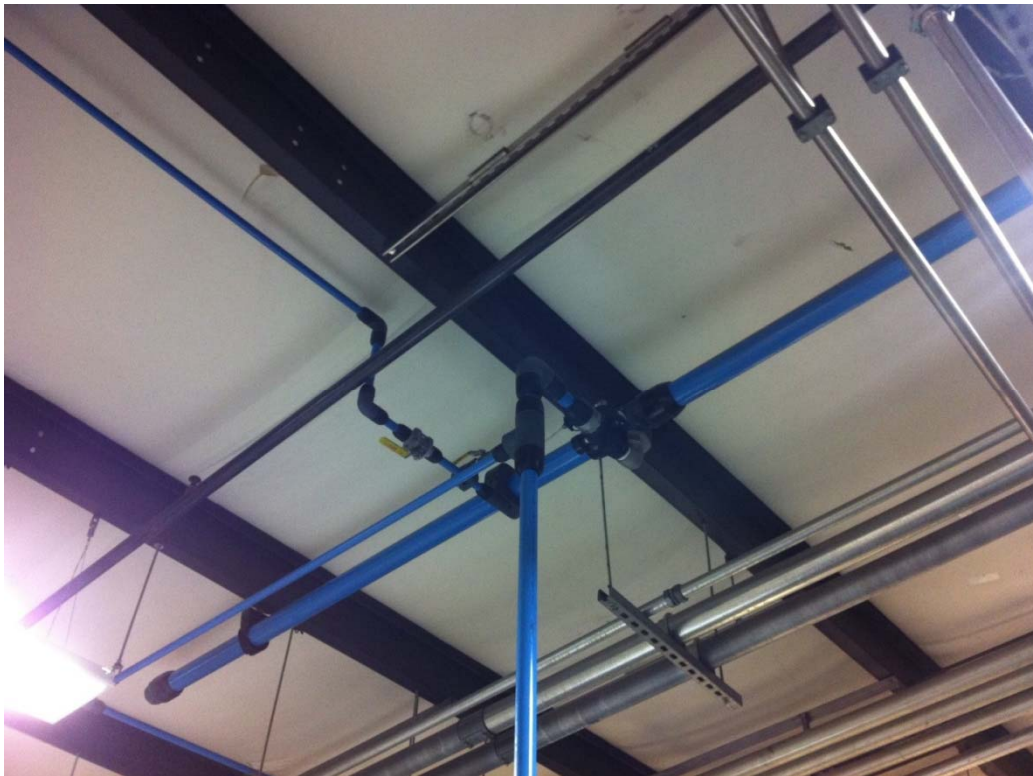
Figure 2-3: Aluminum piping system. Aluminum pipes are blue in color and slip fit connectors are black. Photograph by A.C. Harding, used with permission.
