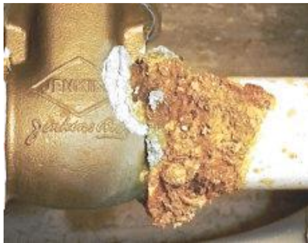
Figure 4 Galvanic corrosion in the connection of carbon steel pipe and brass valve (Courtesy CorrView International Inc.)
