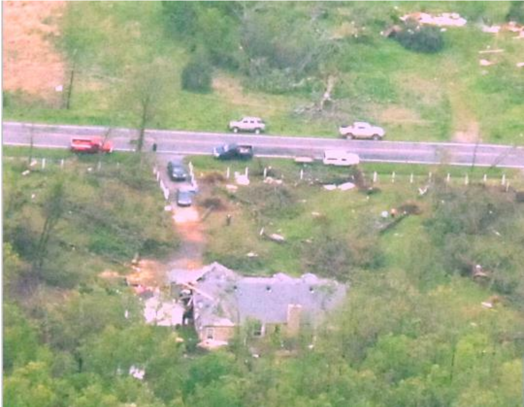
Figure 5.20 Minor damage to the residential house roof rated as EF1, R3L1 taken by CAP (2014).
