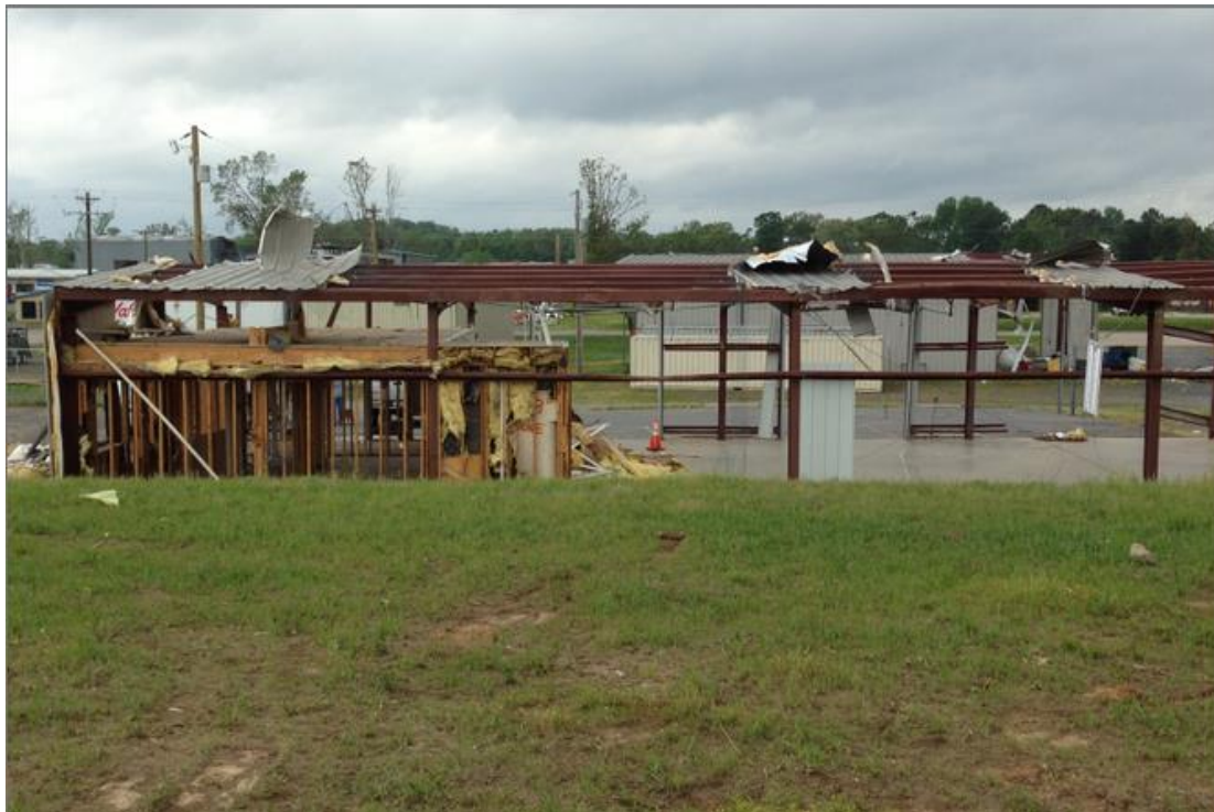
Figure 5.16 A metal at location (R2L3) harshly damaged, almost all the sheets are detached and many columns and beams are bent, Taken by UA team.
