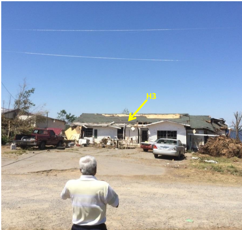
Figure 4.22 Minor damage (EF1) for the house (H3) on the leeward side (low elevation) (UA team photo).
