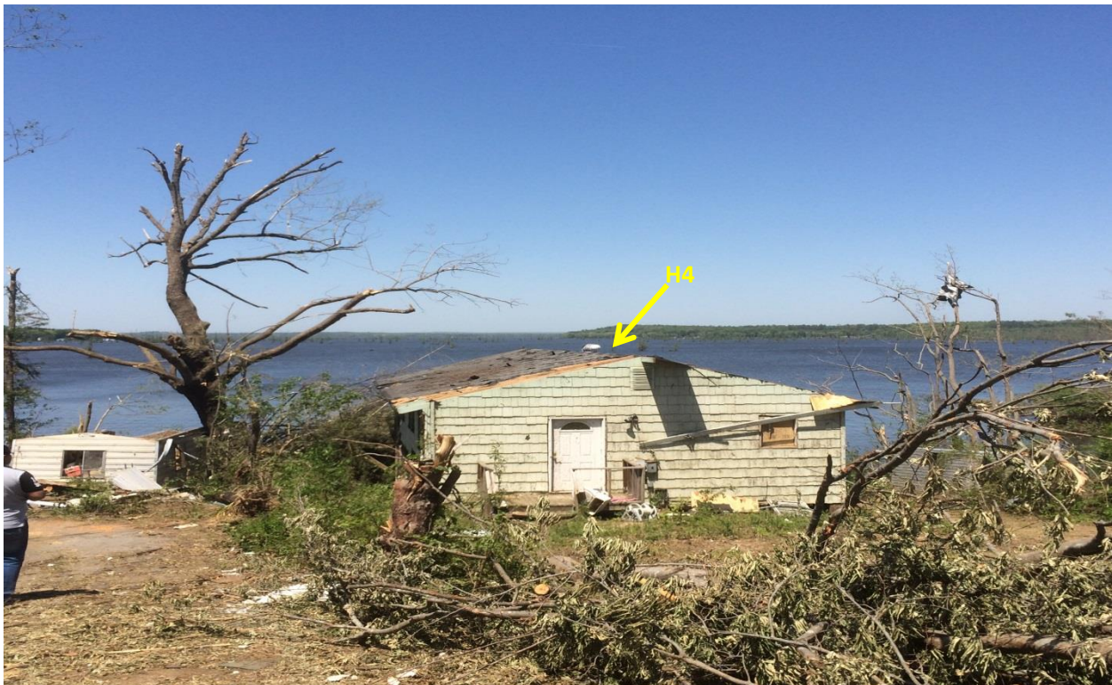
Figure 4.23 Minor roof damage (EF1) for the house (H4) on the leeward side (low elevation 83.8 m (275 ft)). (UA team photo).
