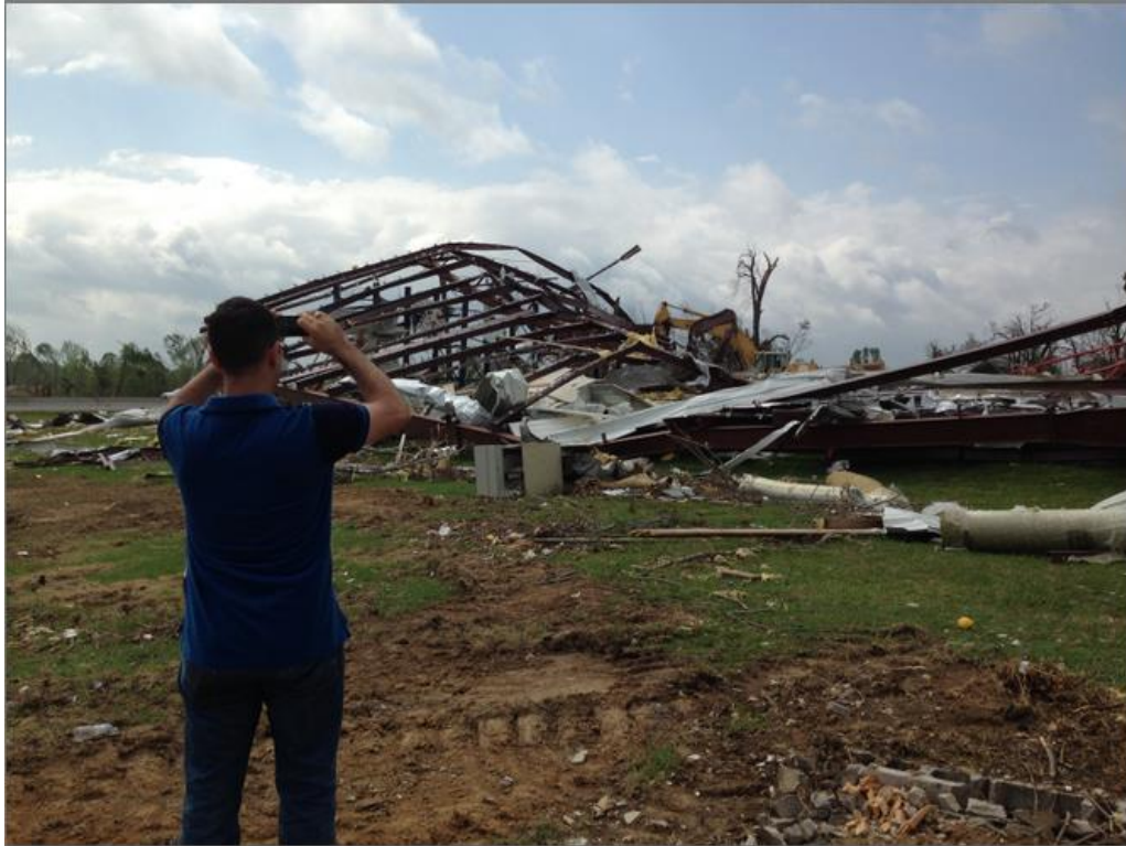
Figure 5.15 A ground photo for a metal building severely destroyed and rated as EF4 at location (R2L3), Taken by UA team.
