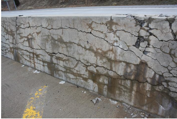
Fig. 1.1-1 –Typical deterioration in concrete barriers due to F/T and ASR (by Richard Deschenes Jr.).
