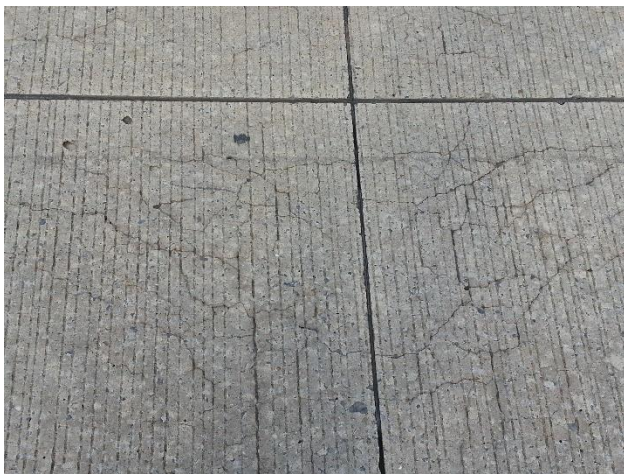
Fig. 1.1-2 –Typical deterioration in concrete pavements due to F/T and ASR (by Richard Deschenes Jr.).
