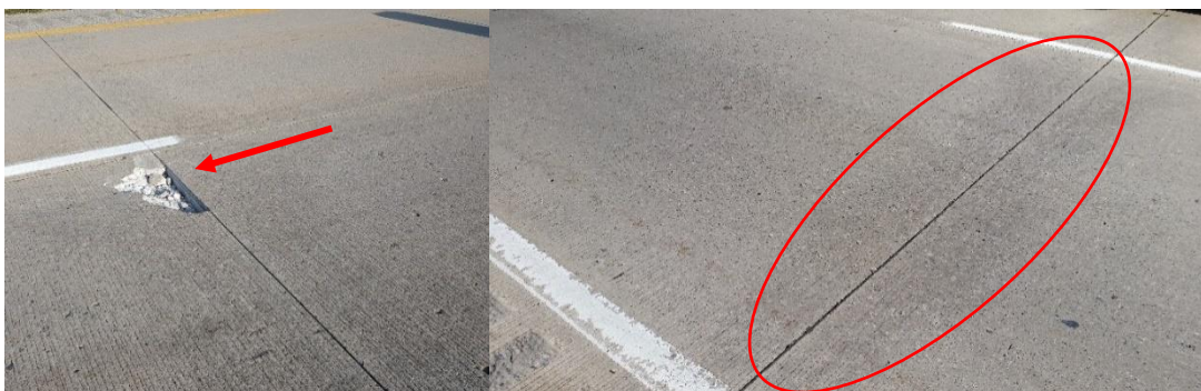
Fig. 4.5-3 –Joint spalling (left) and discoloration (right) (by Richard A. Deschenes).
