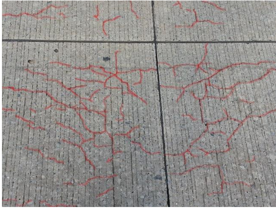
Fig. 5.1-1-D-Cracking in concrete pavement, Interstate 49 (by Richard Deschenes Jr.).
