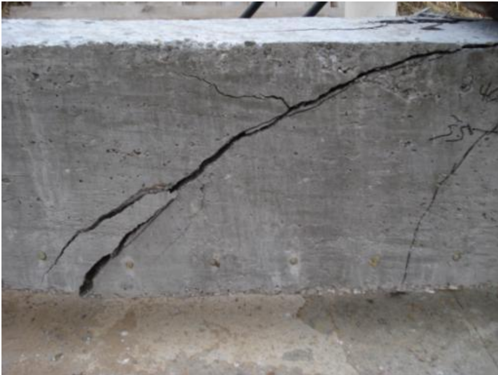
Figure 3-3. Shear/End-Slip failure of NSLS-3D (Photo by author).
