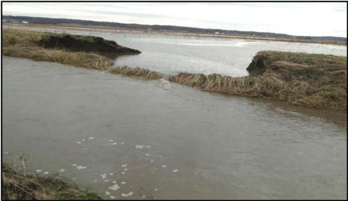
Figure 3 - overtopping erosion in a levee west of Oakford, IL (Rutherford et al., 2016)
