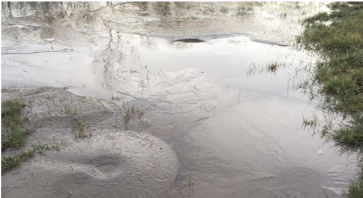
Figure 8 - Sand boils approximately 1,200 feet landward of the levee with water still seeping through near Cairo, IL (Rutherford et al., 2016)
