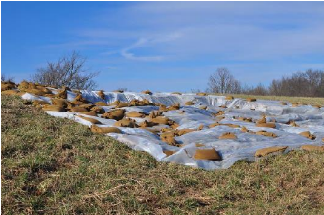
Figure 11 -Surface slide covered with plastic liner and sandbags near Grand Tower, IL (Rutherford et al., 2016)
