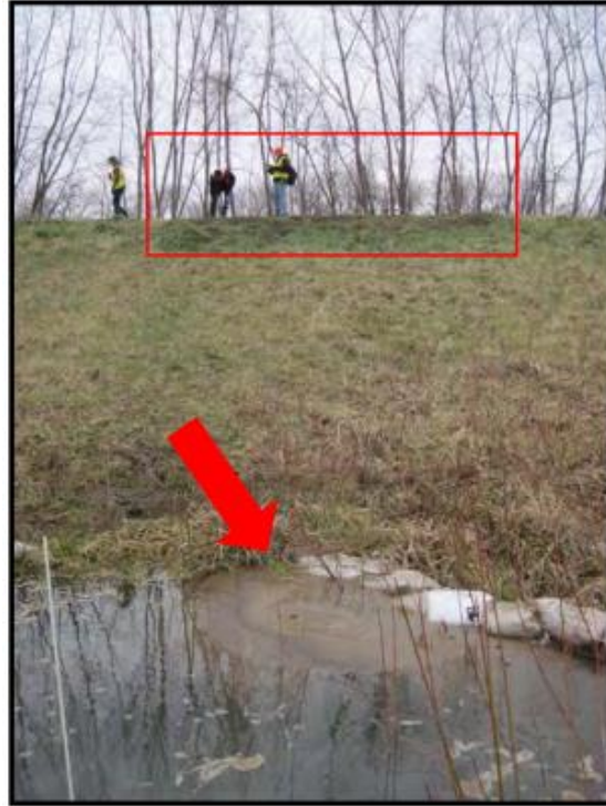
Figure 5 - The arrow indicates the location of a sand boil near the landside levee toe and the box indicates subsidence in levee crest due to loss of soil (Rutherford et al., 2016)
