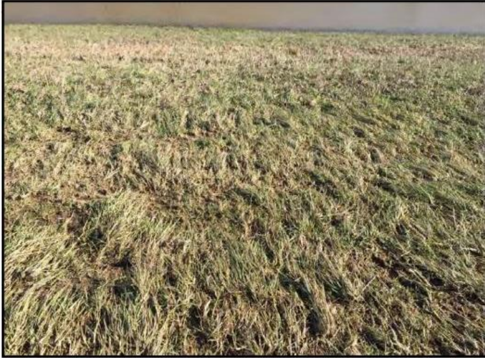
Figure 4 - vegetative cover laid down and acting as an armor on the landside slope of the levee near Olive Branch, IL (Rutherford et al., 2016)
