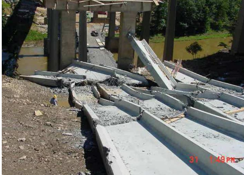
Figure 1.2 - Collapse of I-80 girders in Pennsylvania (Hurff, 2010)
